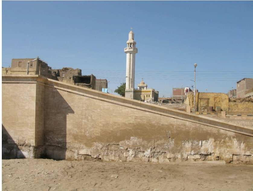
Fig. 8. Accumulation of evaporite salts 1.5 m above the desert surface along the Seti-I Temple outer courtyard retaining wall. Dissolved salts are transported by capillary action. Hieroglyphs within limestone blocks are now almost completely destroyed. Shallow groundwater also is more highly mineralized near these walls reflecting the high rate of localized evaporation.
