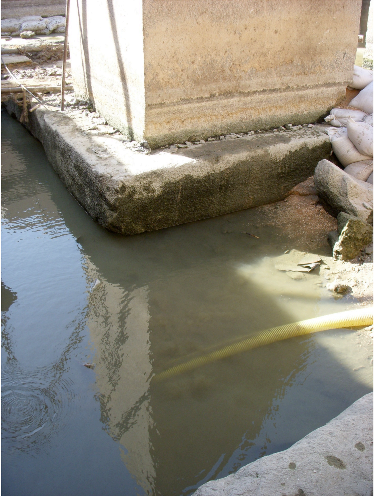
Minimum water level achieved by pumping (view is of column in southwest corner of central island)
