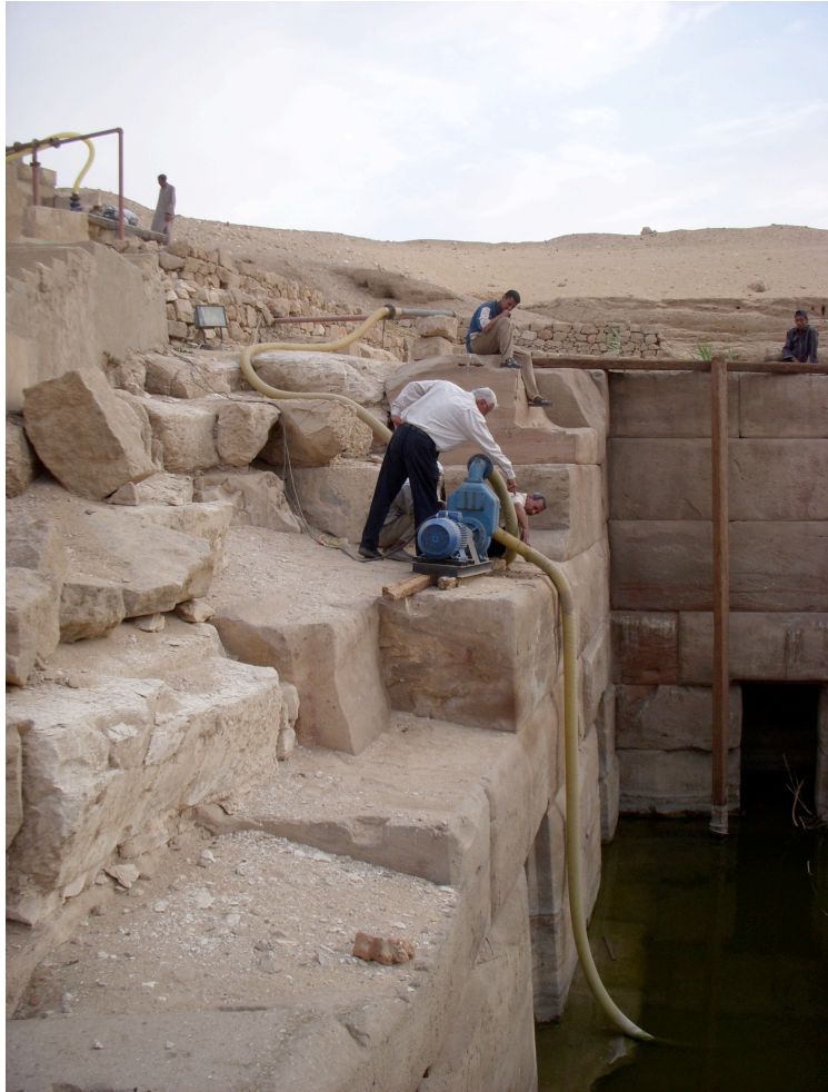
The dewatering pumping set-up (view is towards the southwest corner of the Osireion)
